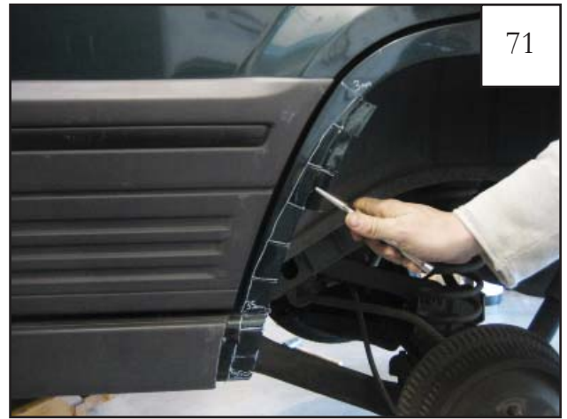
71 Starting at style line, bend cut tabs into wheel well with a heavy hammer. The bend point of the tabs should be on the vertical line drawn in Step 68.
